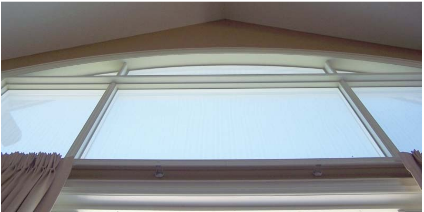
ALL WINDOW UNITS COVERED
